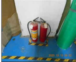
Photo of non-conformity NC Fire extinguishers placed on ground directly.JPG
