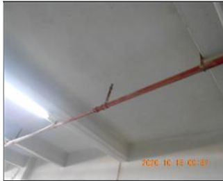
Photo of fire safety equipment Fire sprinkler.JPG
