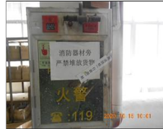
Photo of fire safety equipment Fire hydrant and alarm.JPG
