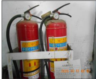
Photo of fire safety equipment Fire extinguisher.JPG
