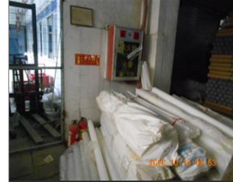
Photo of non-conformity NC Fire hydrant and fire extinguishers blocked.JPG
