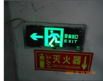
Photo of fire safety equipment Evacuation sign.JPG
