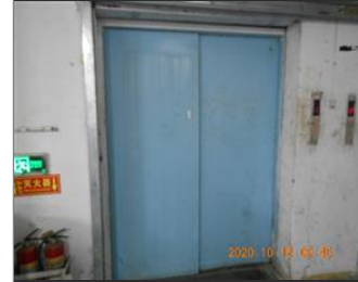
Photo of the inside of the main production hall Cargo lift.JPG
