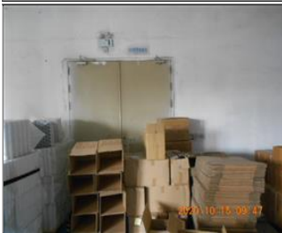
Photo of non-conformity NC Blocked exit 2.JPG
