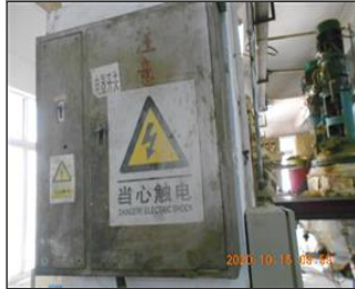
Photo of fire safety equipment Electrical box.JPG
