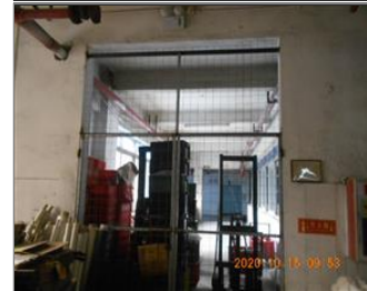
Photo of non-conformity NC Blocked exit 1.JPG
