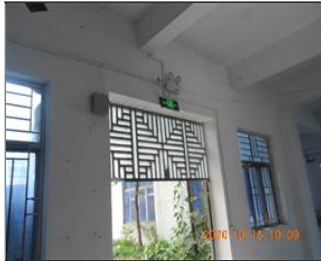
Photo of fire safety equipment Exit sign and emergency light in dormitory.JPG
